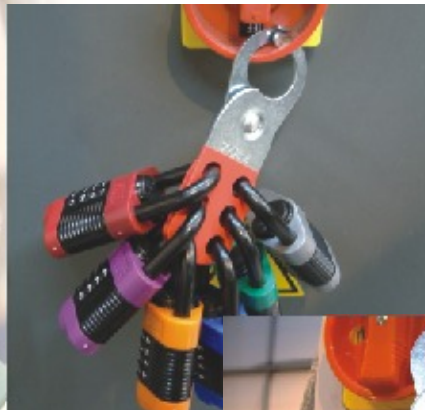
L4 Lock off with Coloured CP1 Padlocks
